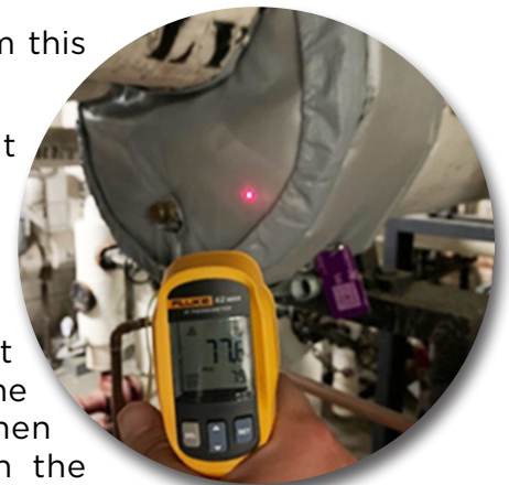
Custom-sized Thermaxx jacket on mechanical equipment.
